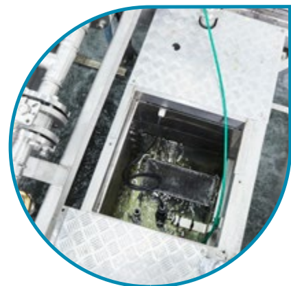
The Taron filter can produce high-quality effluent with TSS less than 10 mg/L.
